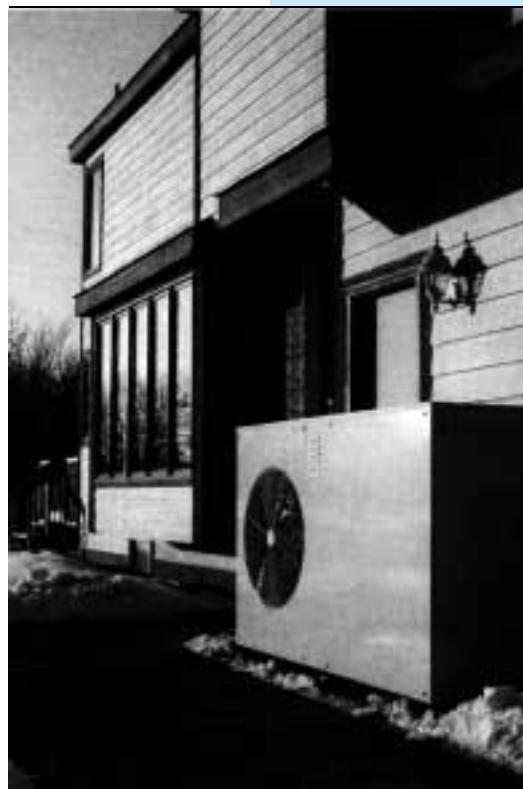
Above: A gas engine-driven heat pump in a residential application.
