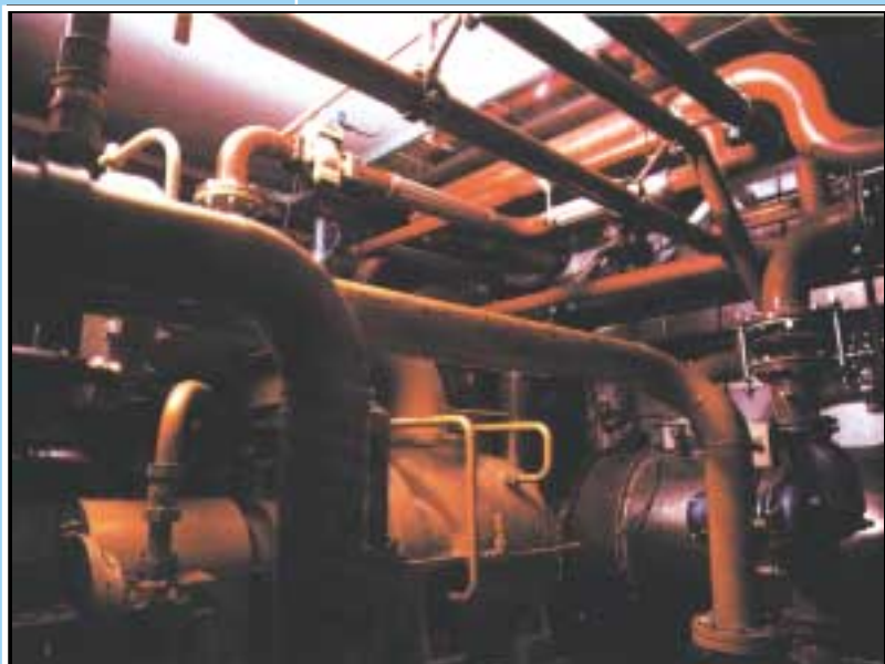
Above: Gas engine driven heat pump for the Amsterdam World Trade Centre.
