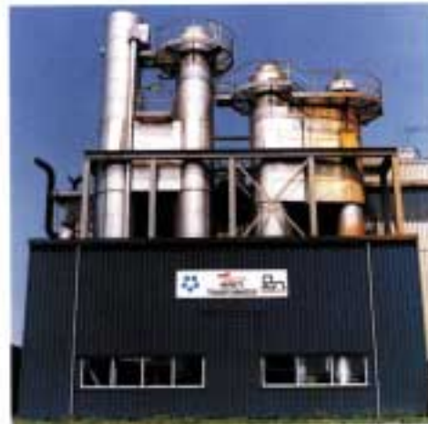
Figure 9 (bottom left): This Absorption heat pump supplies a district heating system using energy from high and low-temperature heat streams from a chemical process.
